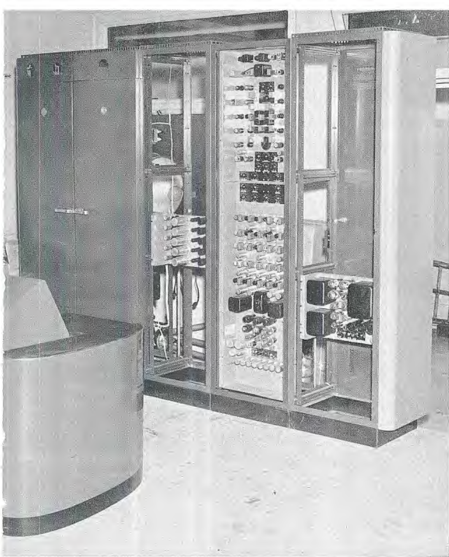
FIG. 3. (left) This photo, taken before installation of equipment was completed, shows the position of equipment racks which are located just behind the control console (a corner of which is visible). On these racks are mounted the main synchronizing generator, monoscope camera, distribution amplifier, and power supplies.
