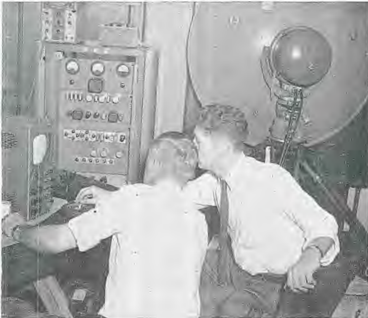
6. Video signal from the microwave transmitter was picked up by this RCA Microwave receiver located in the Lexington Building in downtown Baltimore. The output of this receiver fed the A. T. & T. coaxial cable to New York and Washington.
