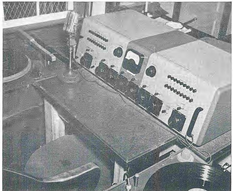
FIG. 8. Turntables are located in the control room as shown here, since there was no room for a separate announce booth. Microphone shown can be used for eüher talkback, or announcing.
